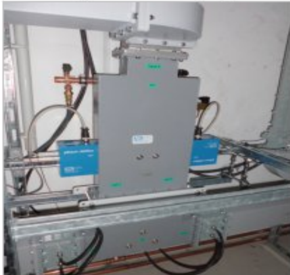
Fig. 1.1 design and manufacturing of the power divider (high energy) and RF phase shifter
